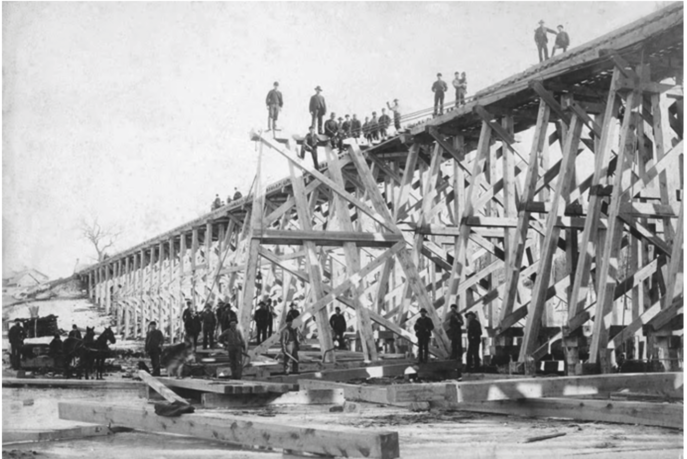
A steam donkey helped to lift the next bent to where it could be slid into place. There were four trains a day here, two freight and two passenger. There were enough hours in between each train so that the workers had time to install the next bent. The line was never closed to trains. In this photo, the workers along with some family members have turned out for photos of one of the bents going in.
